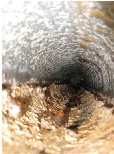
Evidence of trapped water in piping
