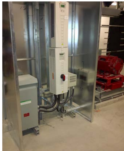
Lineator AUHF and VSD on chilled water pump
