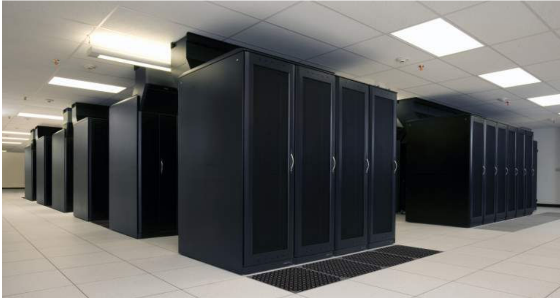
Figure 10: Passive cooling infrastructures use chimneys to contain and recirculate exhaust air
