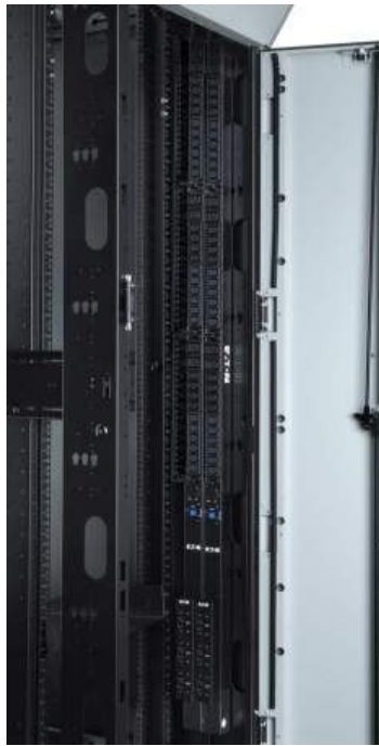
Figure 4: An N+1 configuration like this requires far less space than a 2N architecture, yet still provide adequate redundancy for most purposes.
