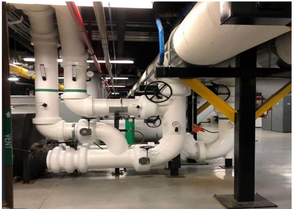
Figure 6 Economizer Piping Modified Installation Photo
