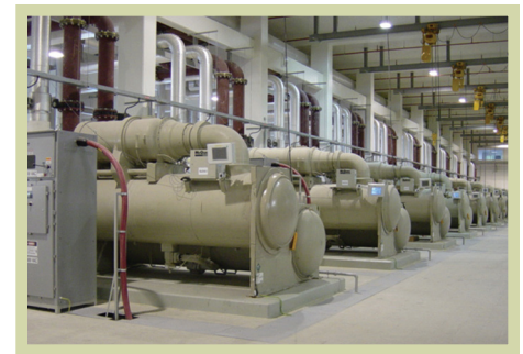
Traditional centrifugal chiller plant
