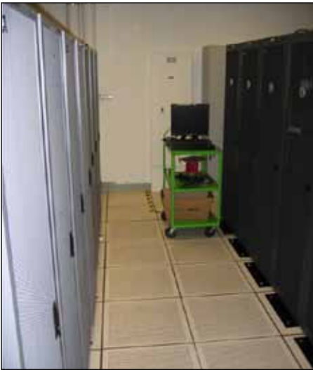
Figure 10: Cause for unusual temperature profile discovered.
