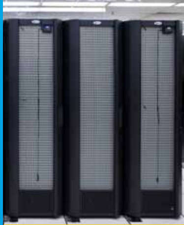
Figure 1: Wireless temperature sensors at LBNL.
