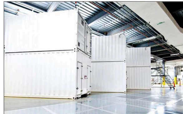
Figure 3: A Chicago Area Data Center Featuring Stacked Container Units
