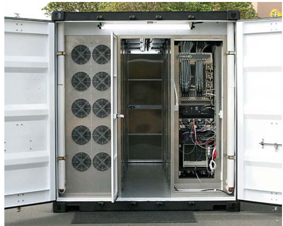
Figure 5: Oracle Sun Modular Data Center, Featuring a Unique IT Rack Layout
