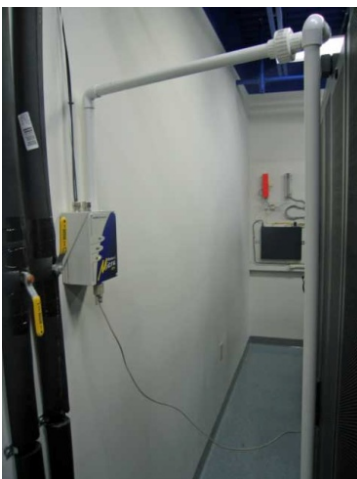
Picture 2: Stratos-Micra 25 with air sampling pipe installed in the return air stream of the CRAC unit
