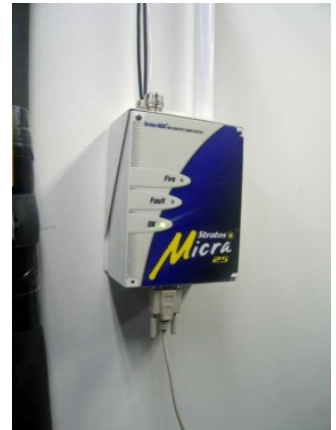
Picture 1: AirSense Stratos-Micra 25 installed
