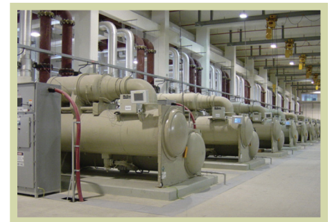
Traditional centrifugal chiller plant
