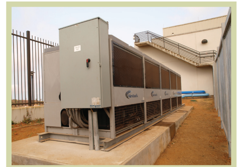
Modular chiller plant
